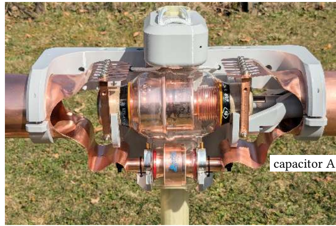
Figure 35: Configuration for 60 m: capacitor A 500 pF is electrically connected. The side screws press the copper tabs onto the capacitor end caps.
